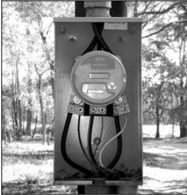
Fig. 1–18. A meter installed in an exterior meter box. (Photo by Landis+Gyr.)
