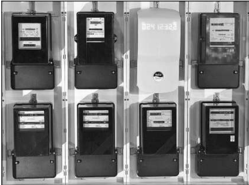
Fig. 2–1. Example of electromechanical meter registers versus a modern customer display unit. (Photo courtesy of Yello Strom.)
