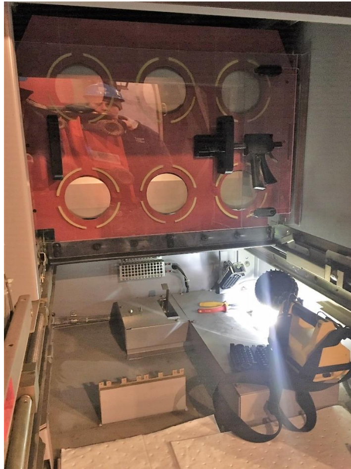
Photo of the Cubicle Inspection & Repair Safety Device Installed at Granite Hill Substation Figure 5
