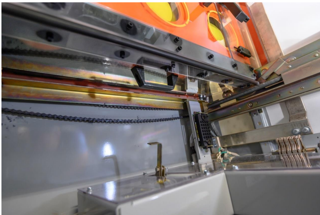
Photo of the Cubicle Inspection & Repair Safety Device Installed (Training Cubicle) Figure 4
