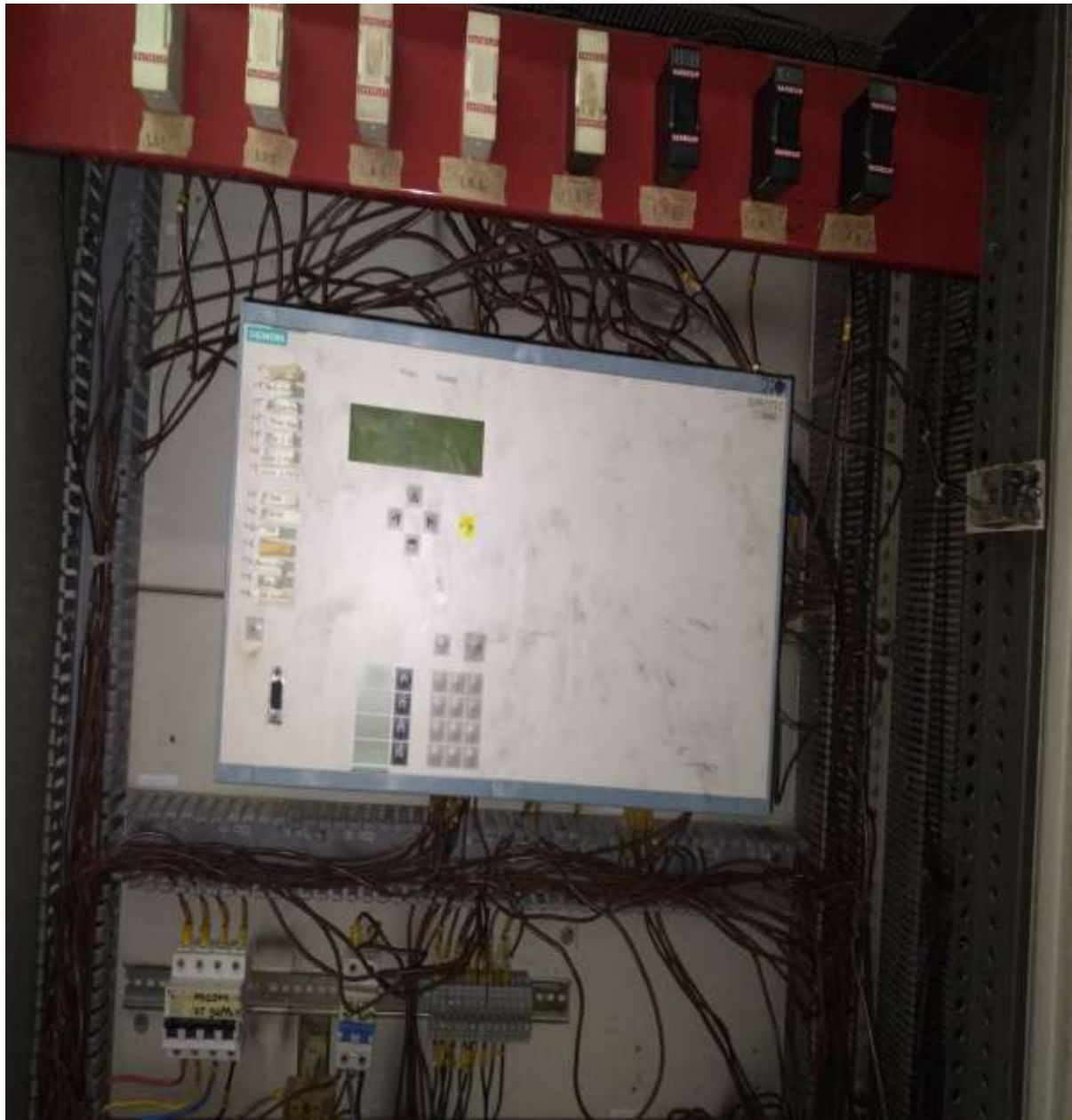
Figure 4: The decommissioned faulty SIEMENS 7SA522 relay
