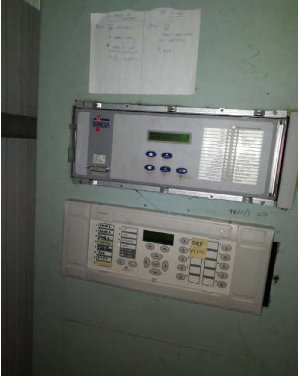
Figure 5: The commissioned MICOM P443 relay
